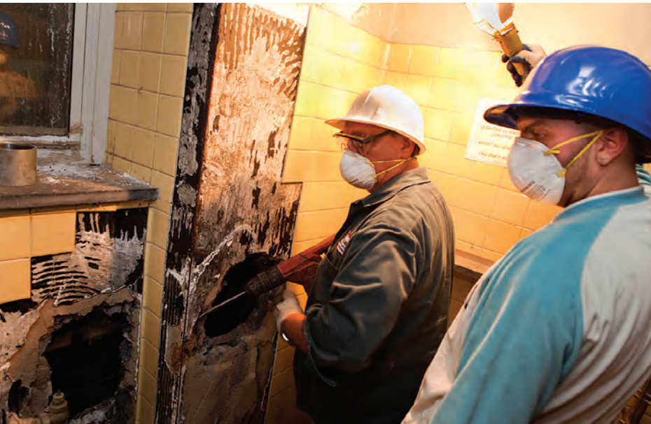
Anthony Mazzacane and Thomas Rea (r.) do major repairs including plaster and tile work at Jacobi Hospital.
